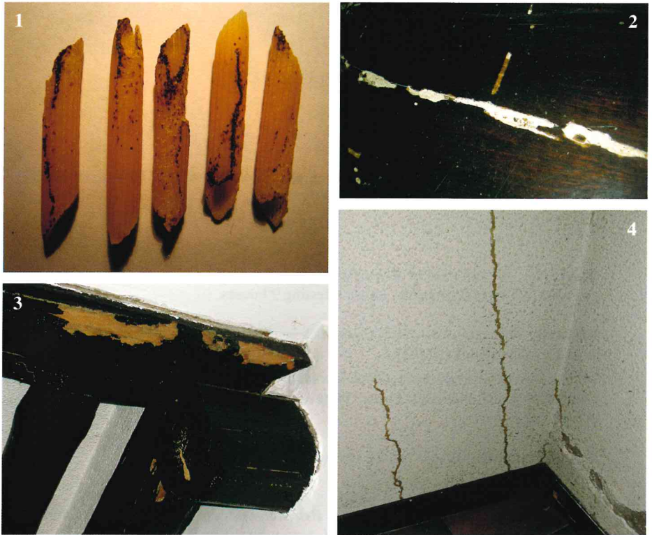
Fig. 1-4: 1, Infestation of Reticulitermes lucifugus on pasta; 2, Damages of R. lucifugus on wood flooring, after uplift and removal of the stair-carpet; 3, Evidence of termite damage to wooden beam, with hanging tubes; 4, Mud tubes constructed by termites on the internal wall of house.
