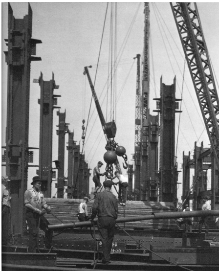
This derrick gang is moving a heavy load of planks while men in the foreground extend the bull-stick of the derrick for greater leverage. Opposite, another connector goes aloft.
